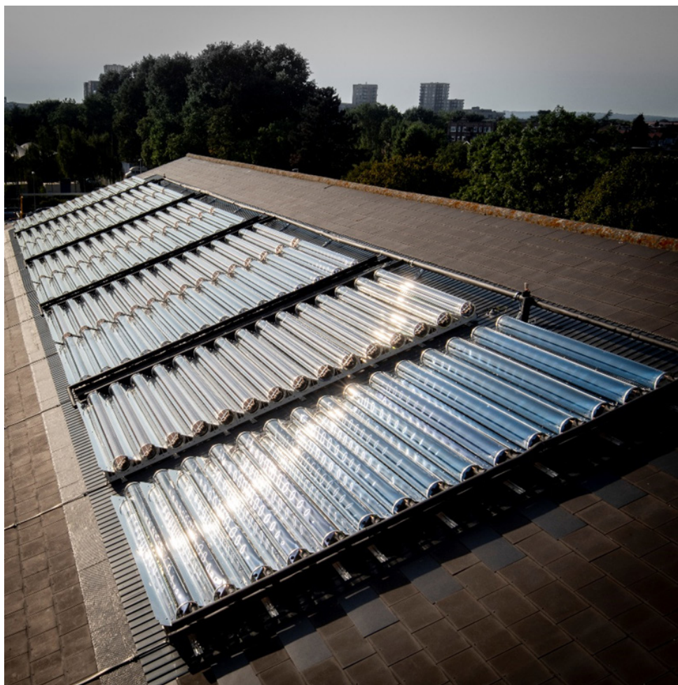
Figure 31: Example of a Virtu solar PVT system in-situ, Naked Energy.
